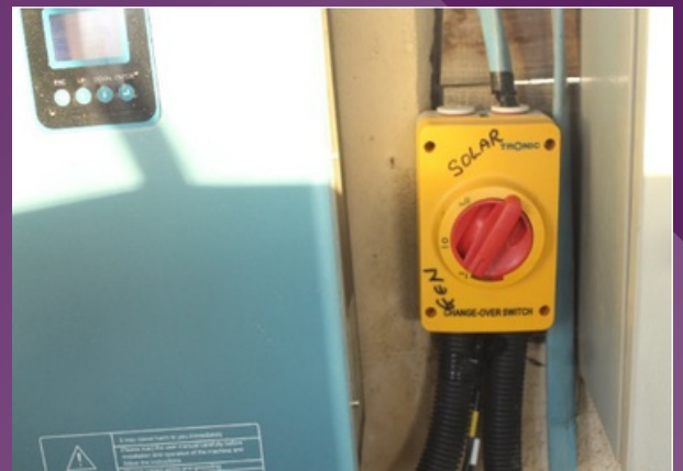
Change-over switch on Shanta abaq hybrid system
